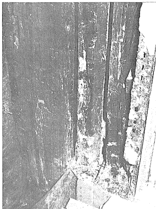
Location: Behind shower stall in 22-year-old home. Cause: No vapor retarder, no bath exhaust, cold outside wall corner.
